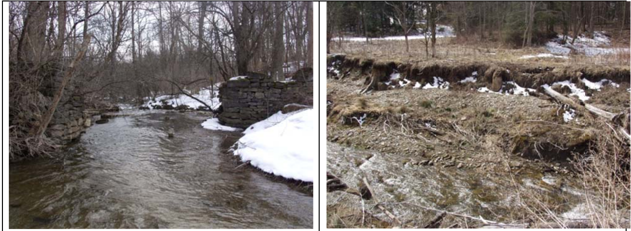
Figure 4: Left, remains of Saw Mill dam near Cassville. Right, remains of a millpond. Note that the stream is cutting through the silt in the foreground and the vegetation is lightly wooded on the former pond embankment in the background.
